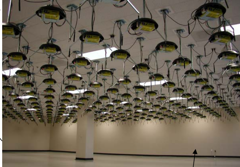
400-node Radio Grid Facility at WINLAB Tech Center
